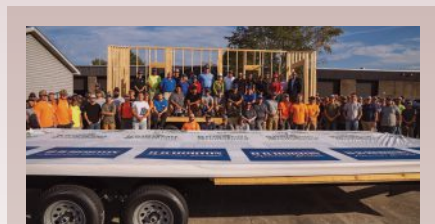
Construction on the homes has begun, with all six schools and the START Center starting on their first tiny homes. Knox County anticipates opening the doors of the village in August 2026.
